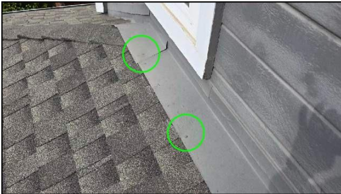
17. Exposed / unsealed fasteners
