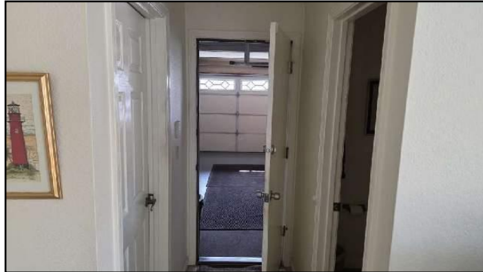
121. Fire door not self closing
