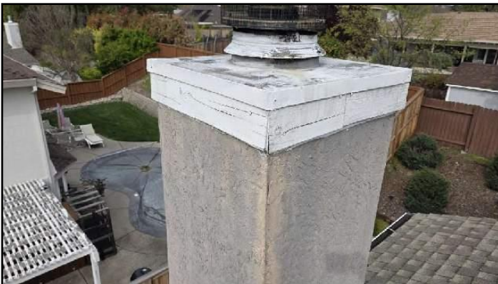
45. Moisture damaged chimney trim boards
