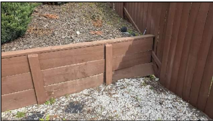
54. Moisture damaged / Leaning retaining wall
