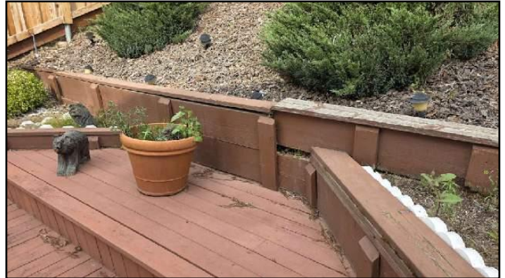
57. Moisture damaged / Leaning retaining wall
