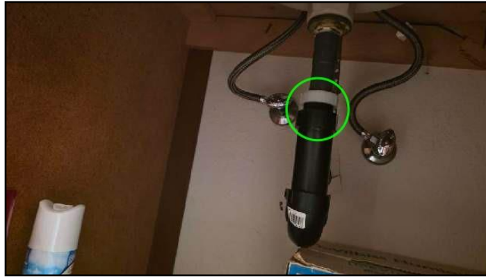
97. Leak at sink drain line
