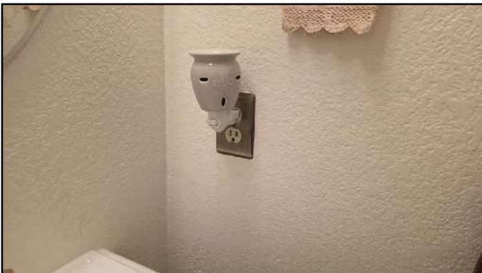
71. Outlet not GFCI protected
