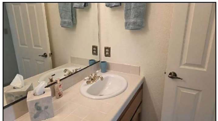
74. Outlet not GFCI protected
