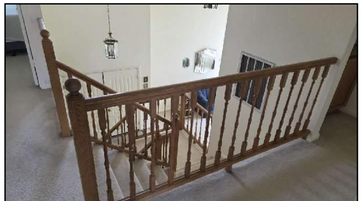
119. Guardrail lower than current standards
