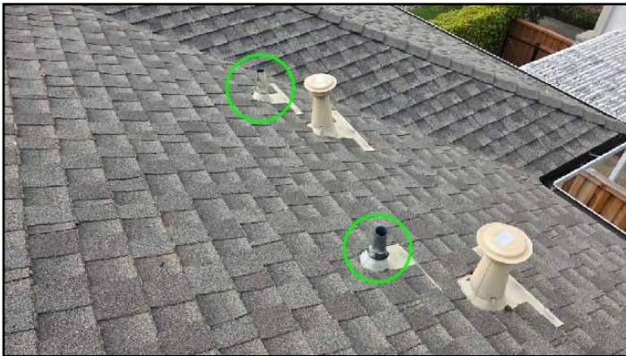
13. Cracked rubber boot collars
