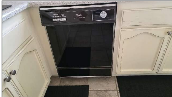
122. Dishwasher missing air gap and high loop
