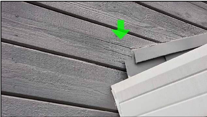
47. Moisture damaged wood siding
