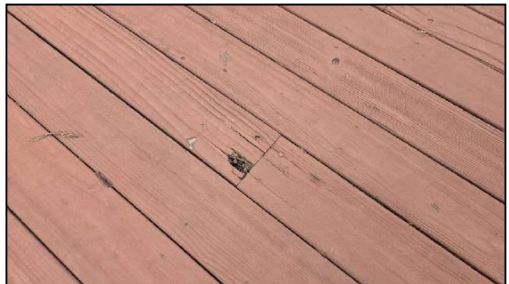
52. Moisture damaged deck boards and framing
