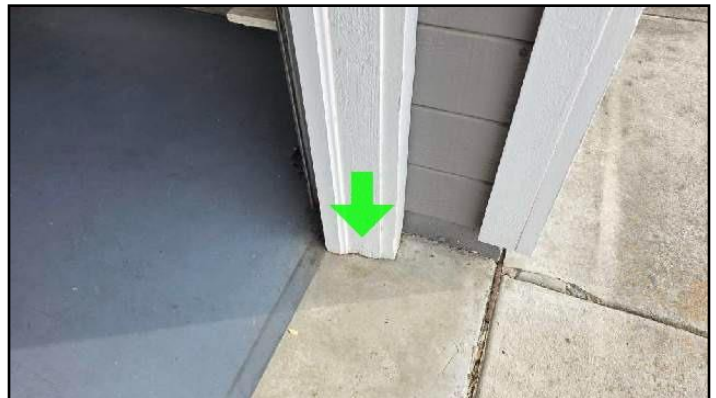
46. Moisture damaged vehicle door frame
