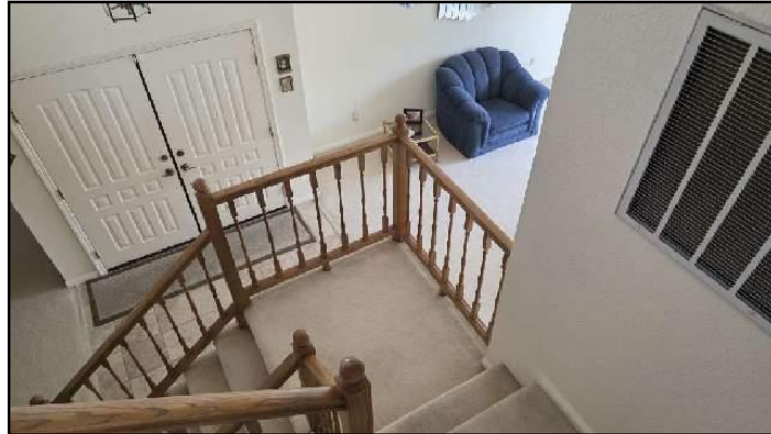
120. Guardrail lower than current standards
