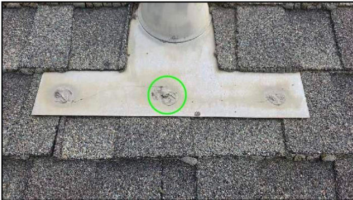
11. Exposed / unsealed fastener
