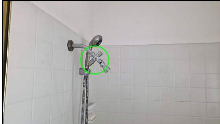
100. Shower head assembly leaks
