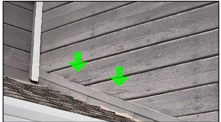
48. Moisture damaged wood siding
