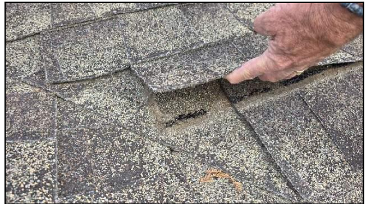
14. Loose valley shingles
