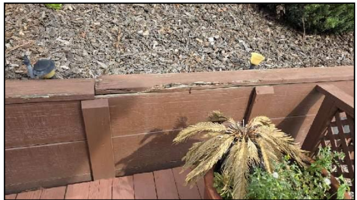
55. Moisture damaged / Leaning retaining wall
