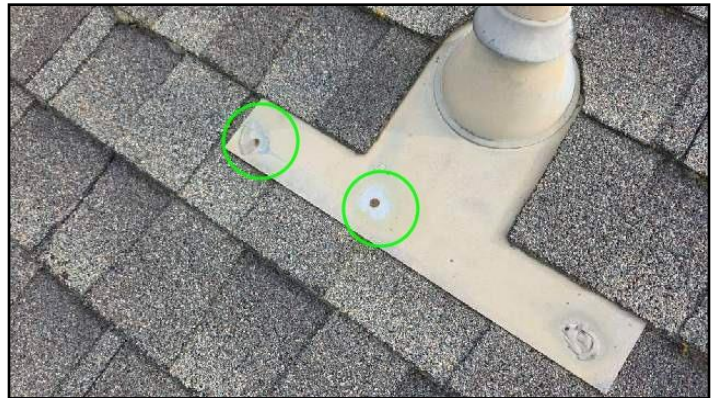
26. Exposed / unsealed fasteners
