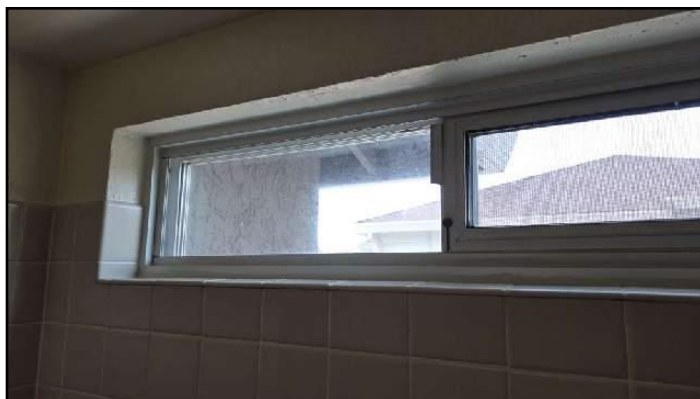
117. Failed window seal
