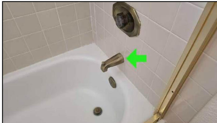
98. Deteriorated tub spout sealant
