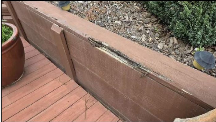
56. Moisture damaged / Leaning retaining wall
