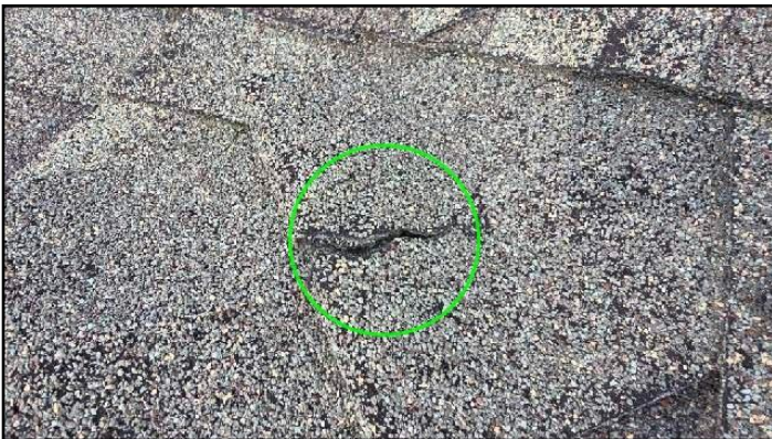
9. Cracked hip shingle
