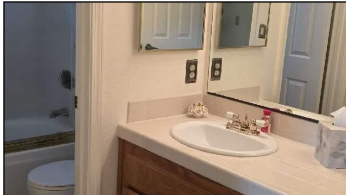
75. Outlet not GFCI protected
