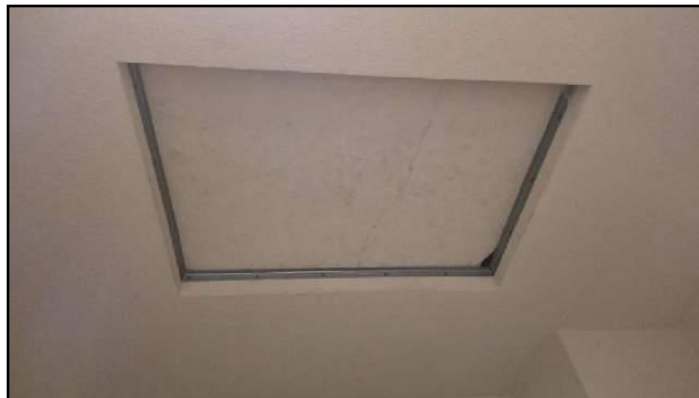
114. Damaged attic access cover
