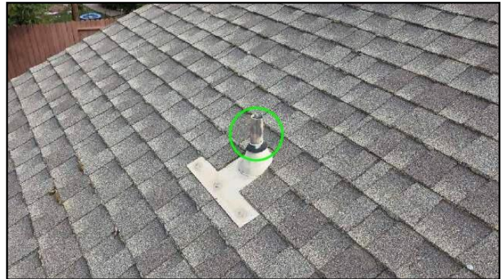
12. Cracked rubber boot collar
