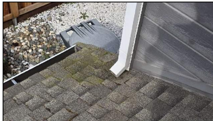
42. Downspout discharges onto roof
