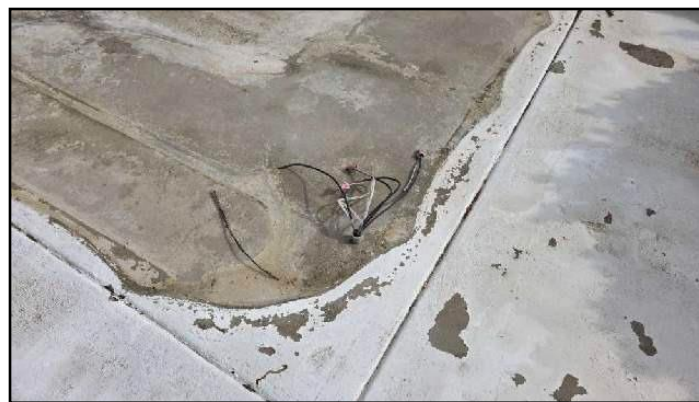
70. Wire ends not contained in a junction box
