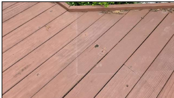
53. Moisture damaged deck boards and framing
