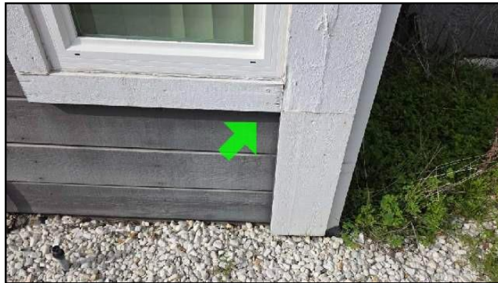
49. Moisture damaged wood siding / trim
