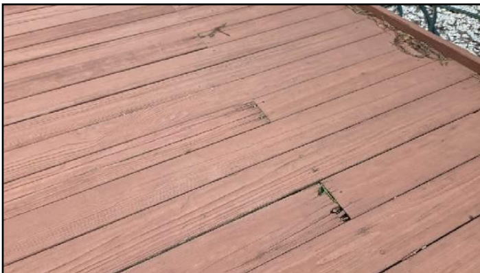
51. Moisture damaged deck boards and framing
